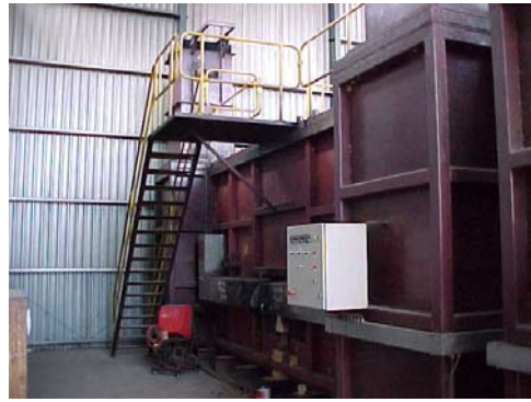
Figure 9: Charcoal Gasification Plant
