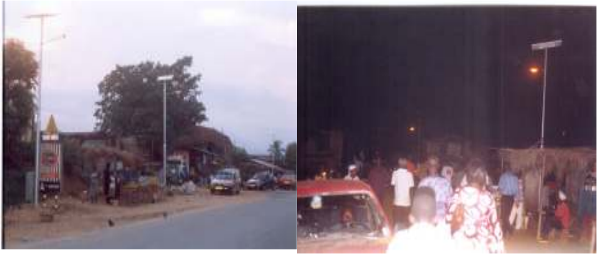
Fig.1: Solar Street Lights installed at Teacher Mante
