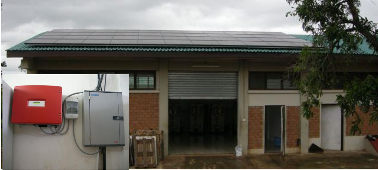
Figure 1: The 4.18 kWp Grid Connected Solar PV System at Pure Company, Benkrom, near Buipe
