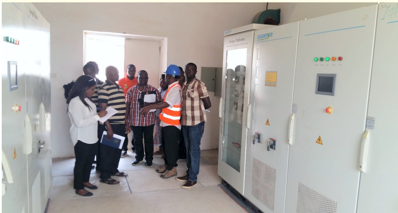
Figure 8: EC Monitoring Team and Site Engineers inspecting the Invertor Room
