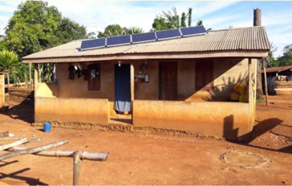
Figure 18 : 500Wp solar PV panel installed in a Rural Household
