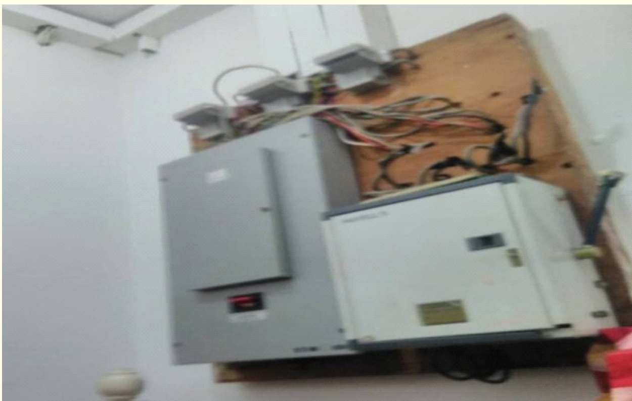
Figure 10: Untidy Cabling and DB not labelled
