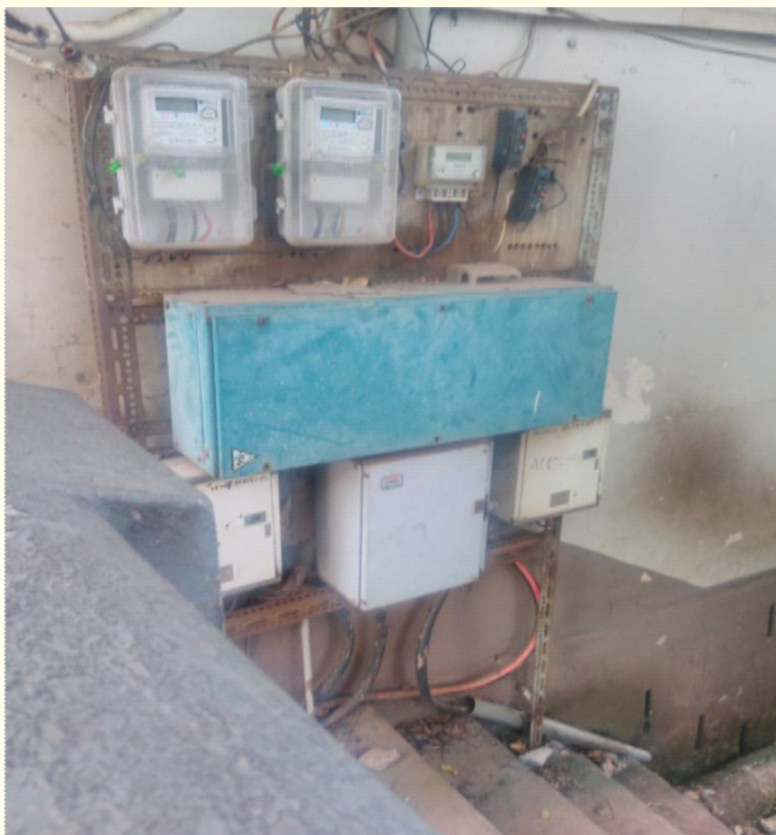
Figure 5: Exposed power board at KMA
