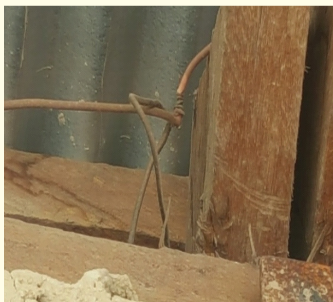
Figure 3: Exposed, live conductor
