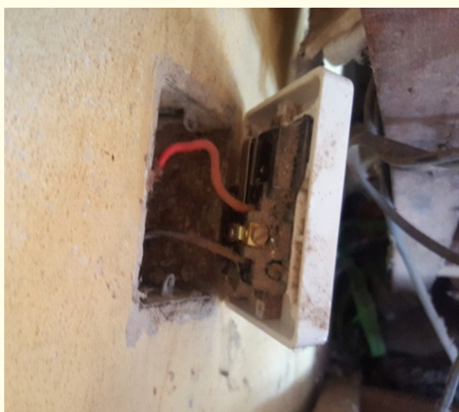
Figure 2: Socket without a circuit protective conductor
