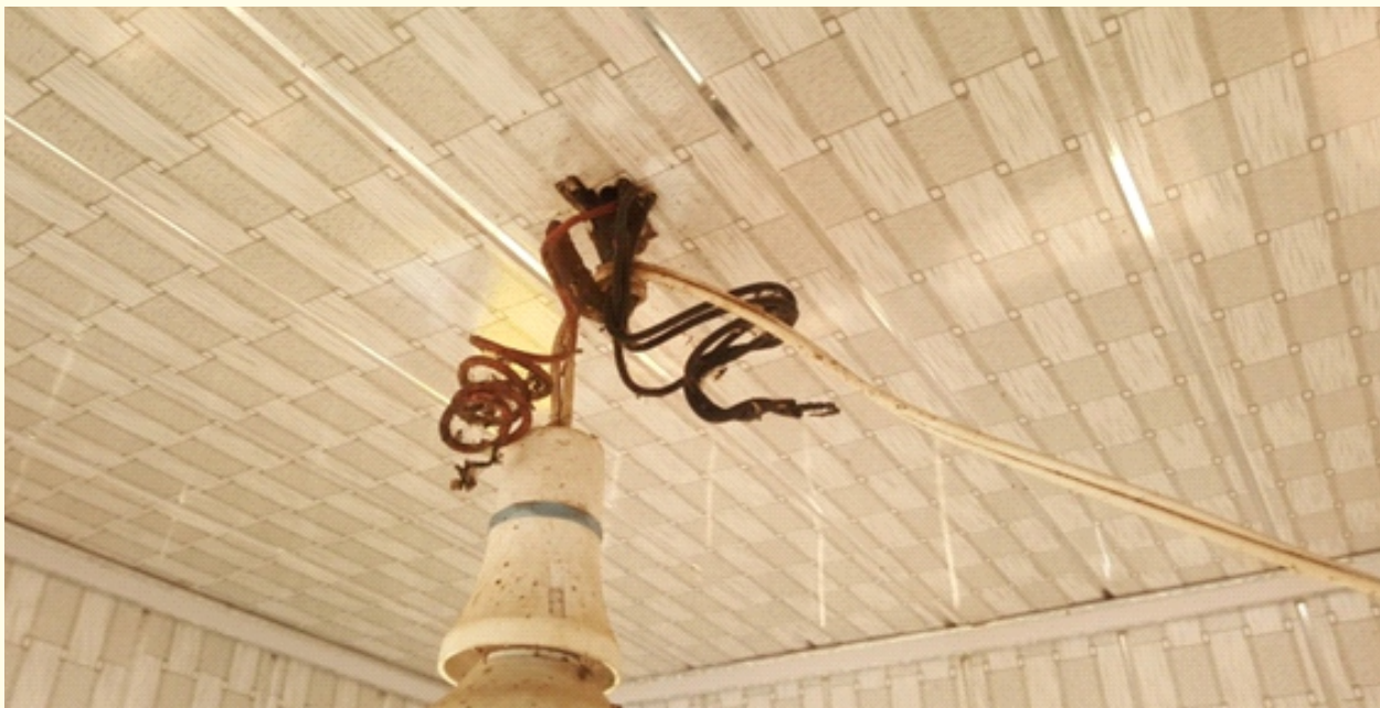
Figure 4: Exposed live cables
