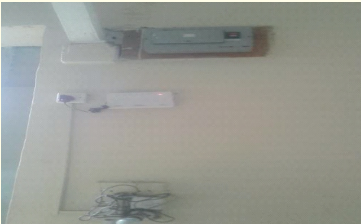
Figure 6: Consumer Units mounted too high
