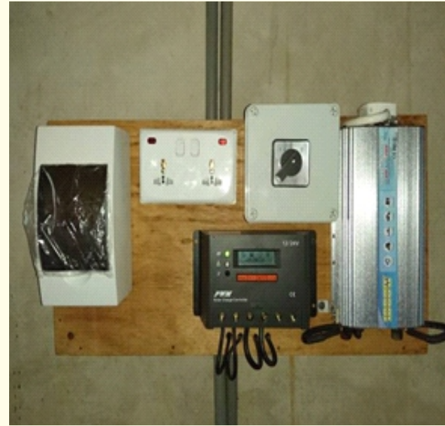
Figure 19: Installed Balance of System (BoS)
