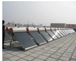
Cloud Thermal Solar Hot Water System
