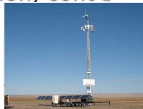
Mobile Solar Powered Platform
