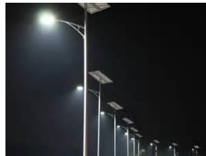
Solar Street Lighting
