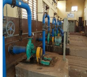
High 3- \phi pumps
