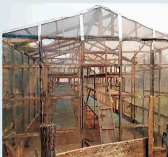
Dilapidated state of the dryer after windstorm
