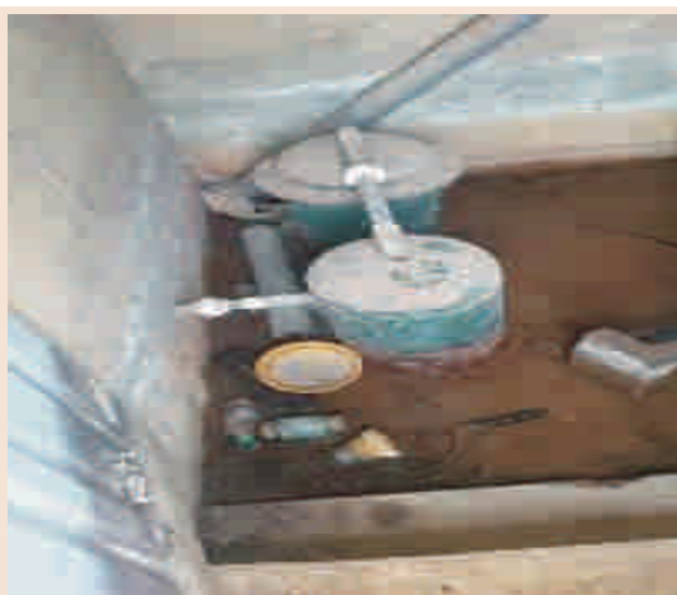
Effluent filtration system for SOS biogas plant
