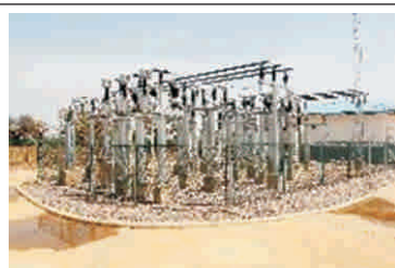
The Plants substation
