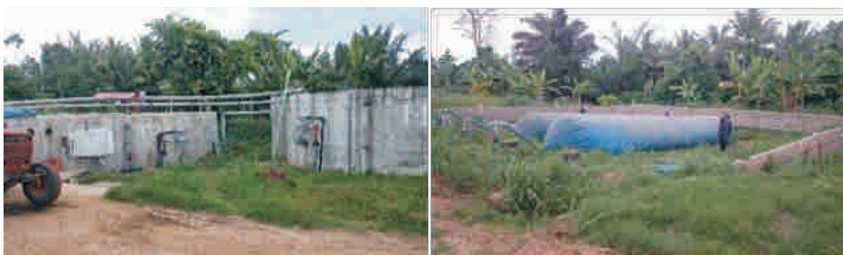
Figure 4: Concrete Digester at HPW Fresh and Dry (Left: Two 450m 3 concrete biogas digesters. Right: Three holding balloons for the storage of the gas)
