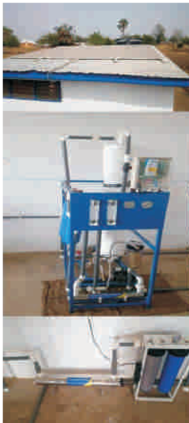
(From top: Solar PV for powering filtration system, Reverse osmosis equipment for water purification, UV and filtering apparatus)
