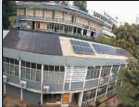
Figure 34: Part of the 44kW solar PV installed at KNUST
