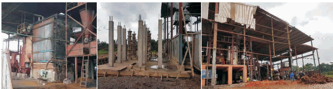
Left: 6t/hr boiler Middle: Civil works for boiler expansion, Right: Preparing palm fruits for processing
