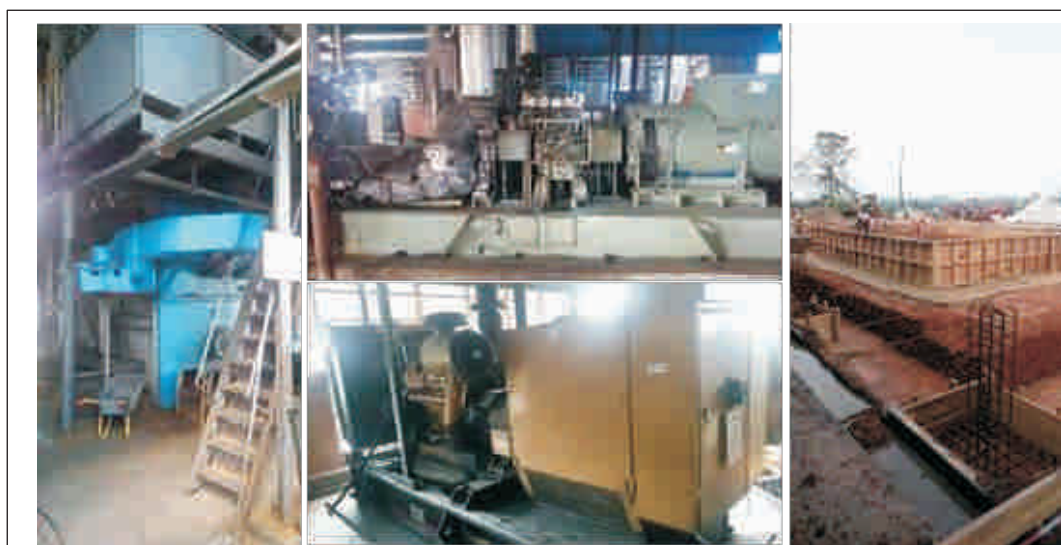
Figure 15: Biomass Cogeneration Plant at Twifo Oil Palm Plantation
