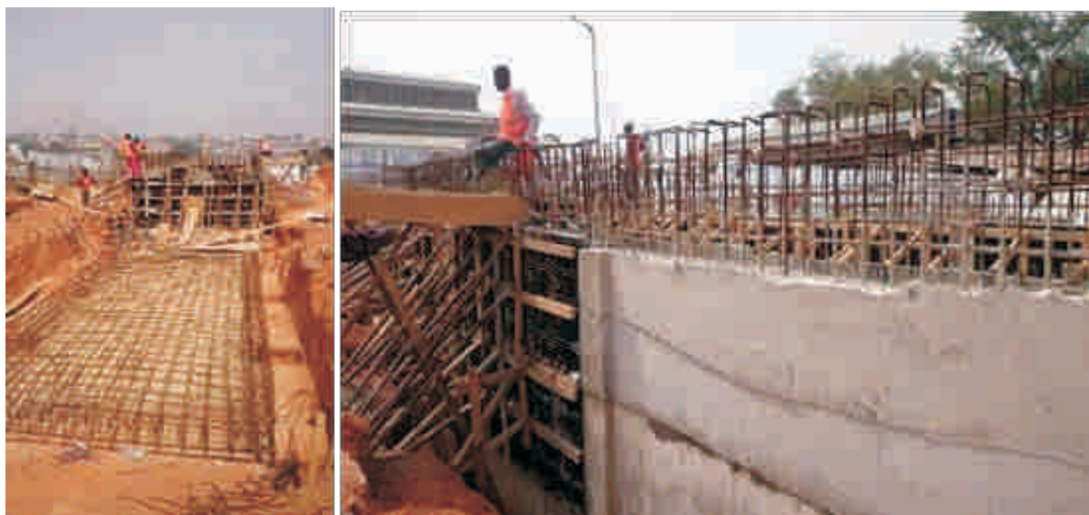
Figure 7: Civil works for a biogas facility under way at the Kumasi Abattoir
