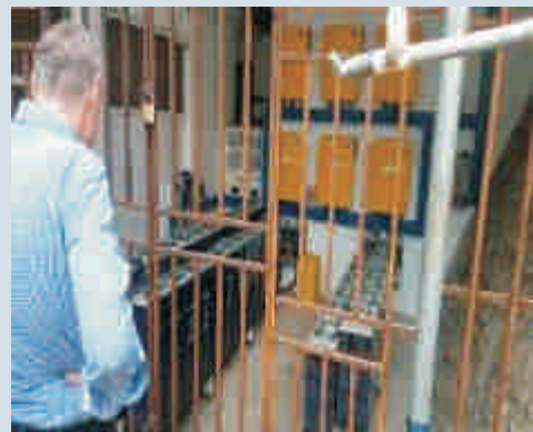
Figure 35: Smart energy management system at KNUST
