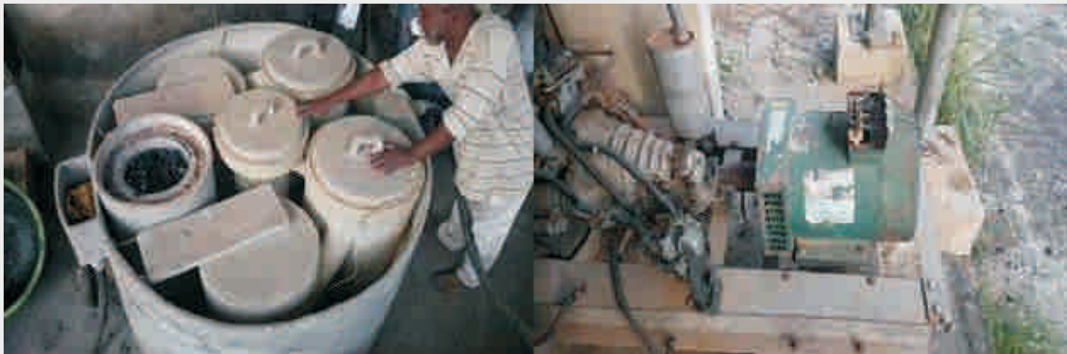
Figure 41: 10kW gasifier plant at TCC
