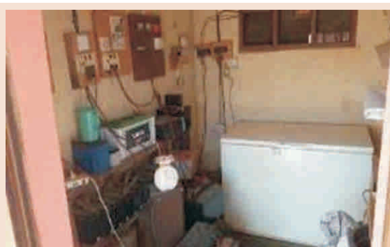
Figure 24: Equipment at the Solar Charging Centre
