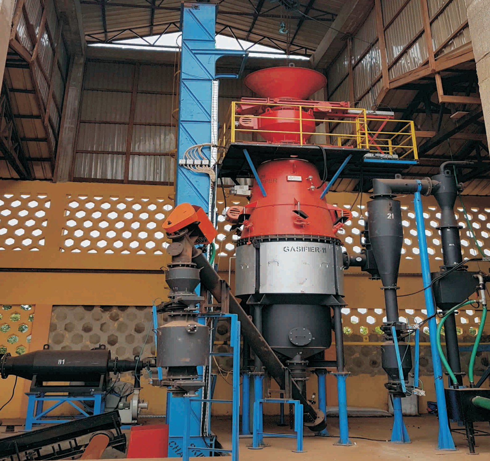
120 kW Gasifier plant installed in Ghana - the biggest gasifier plant installed in Africa
