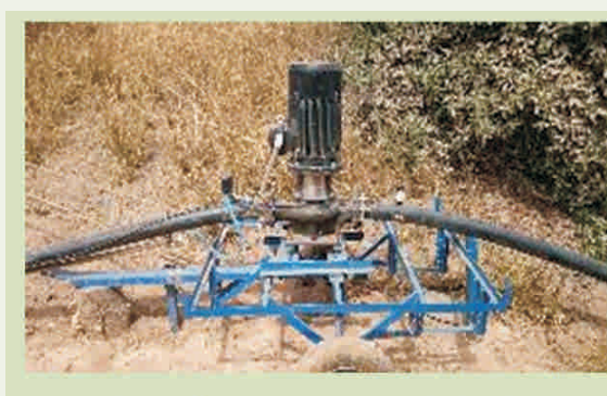
30kw pump for irrigation
