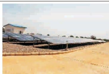
Solar panel array at the plant
