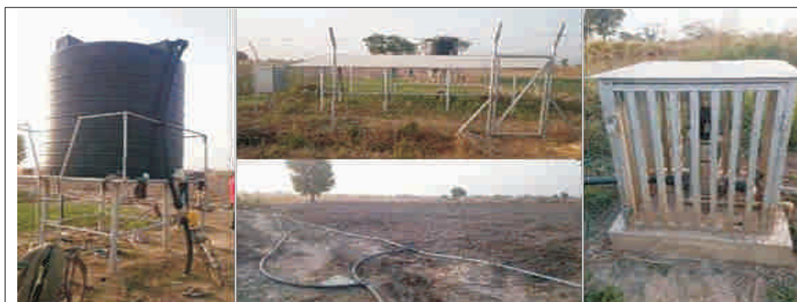
Figure 21: Datoyili solar irrigation set up
