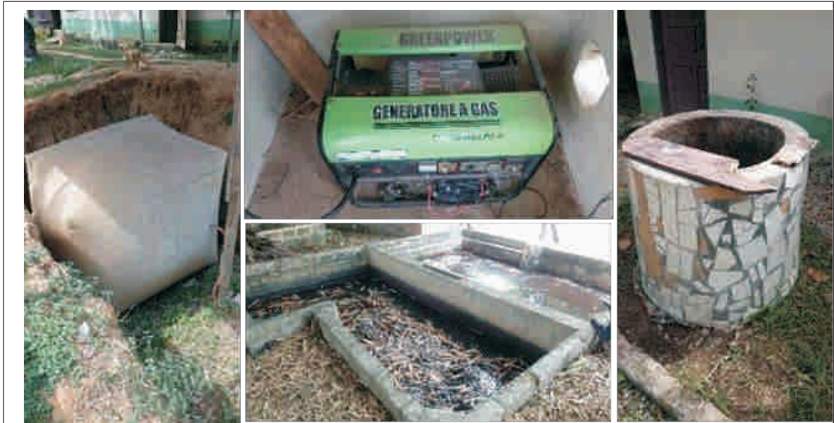
Left: Gas holder. Middle top: 15 kVA biogas generator. Middle bottom: Spent sludge holder. Right: Underground digester head.
