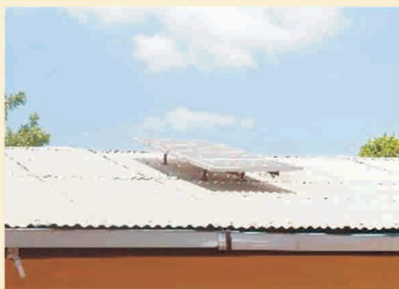
A 100W solar system provided to power a health center
