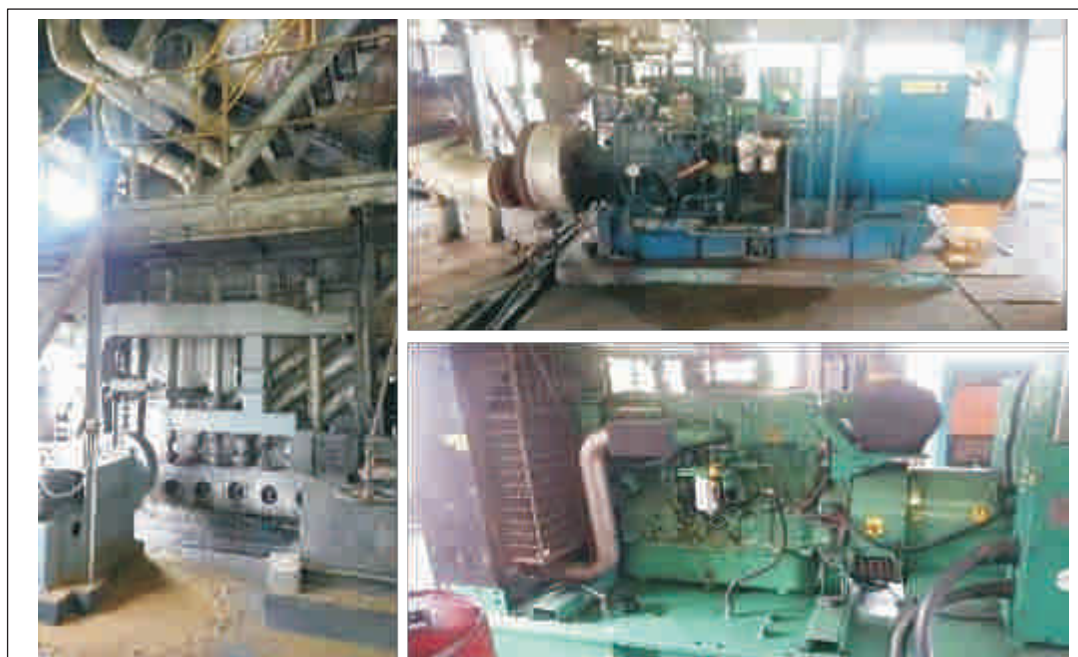
Figure 14: Biomass Cogeneration Plant at Benso Oil Palm Plantation
