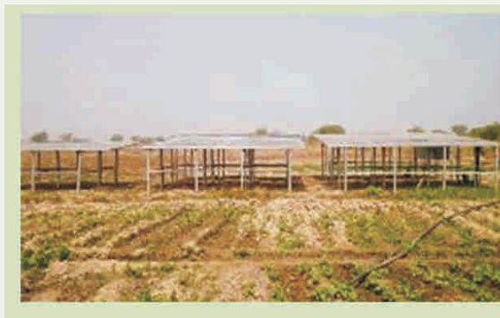
15kw solar PV at Tamalugu
