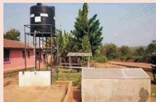
Figure 25: Solar water pump and solar water still installed adjacent the centre
