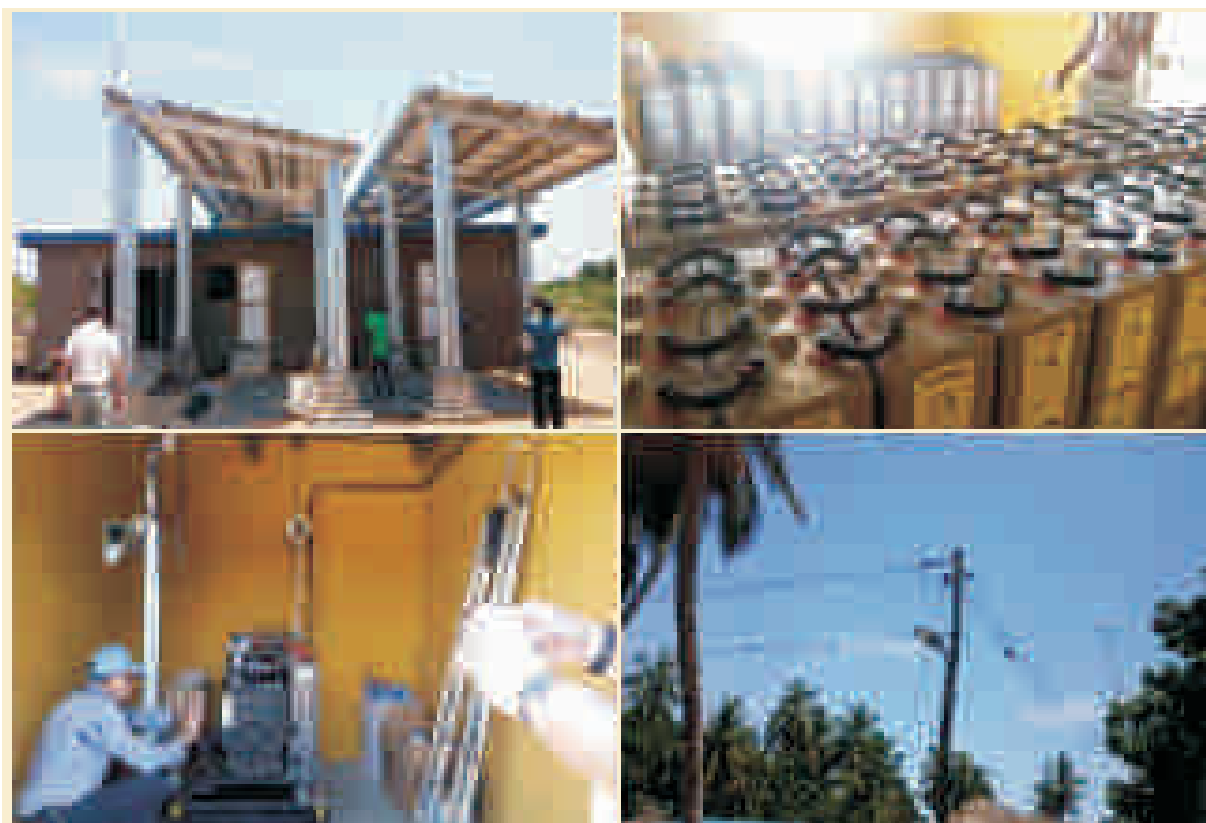
Top left: Solar panels mounted on high metallic structures. Top right: Battery bank for storage. Bottom left: 30kVA diesel generator. Bottom right: transmission lines with LED streetlight
