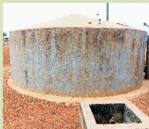
The storage tank provided for the pumped water
