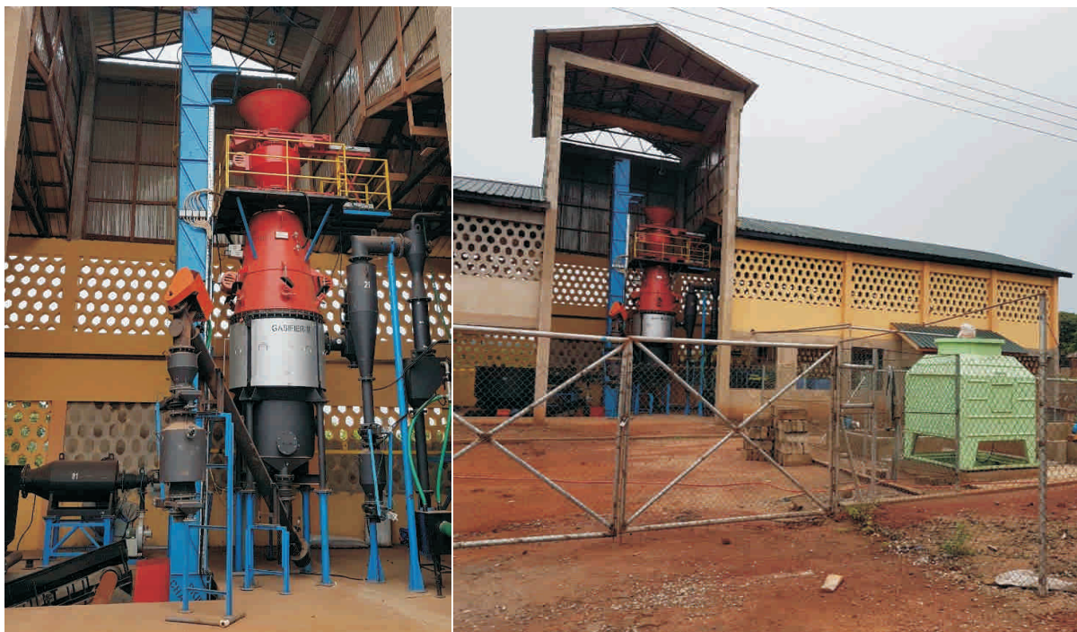
Gasifier with its appurtenance installed in the gasifier house
