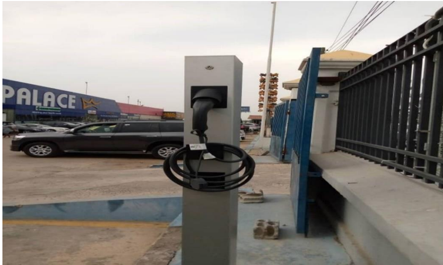
Figure 7: Porsche Charging Station located at Palace Mall, Spintex Road
