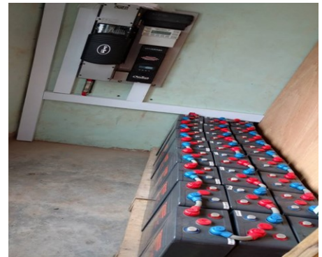
Complete Battery Bank (Photo credit: Power World Ltd.)
