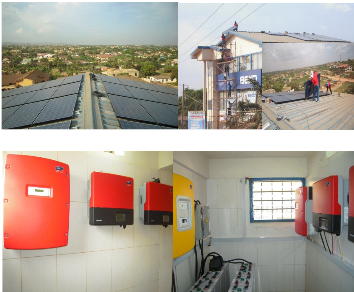
Figure 1: Installation of 10.6 kWp grid connection at the office of Tradeworks Co. Ltd.
