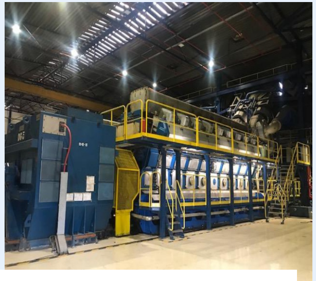
Fig 4: Inspection of Wholesale Suppliers (Powerhouse 3 at Aksa)
