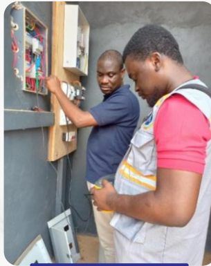
Officers Inspecting and Testing a Facility Owners Consumer Unit at Kpeve during Compliance Monitoring
