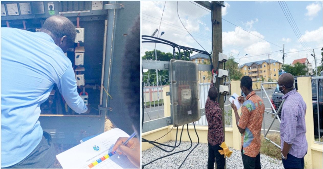
Figure 4: Transformer load monitoring at Nigeria High Commission Substation
