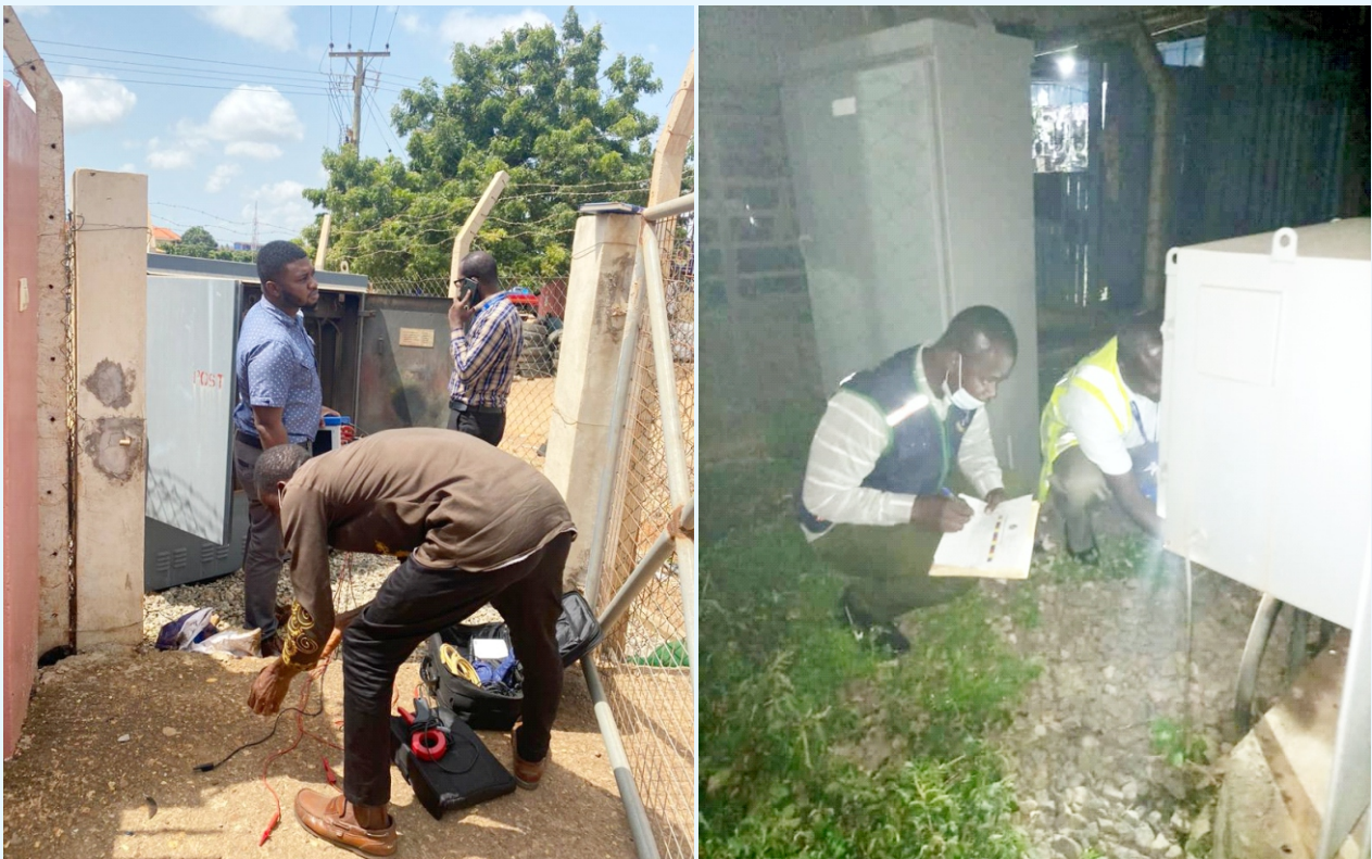
Fig. 5: Installation of power analyzer for power quality monitoring (replace pics)
